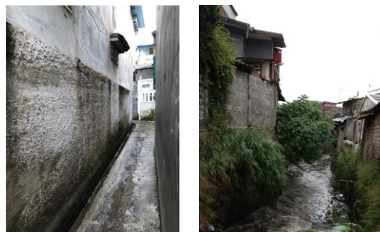
Figure 3. Conventional Drainage System in Cibadak administrative village (Left) and the Citepus River (Right)
